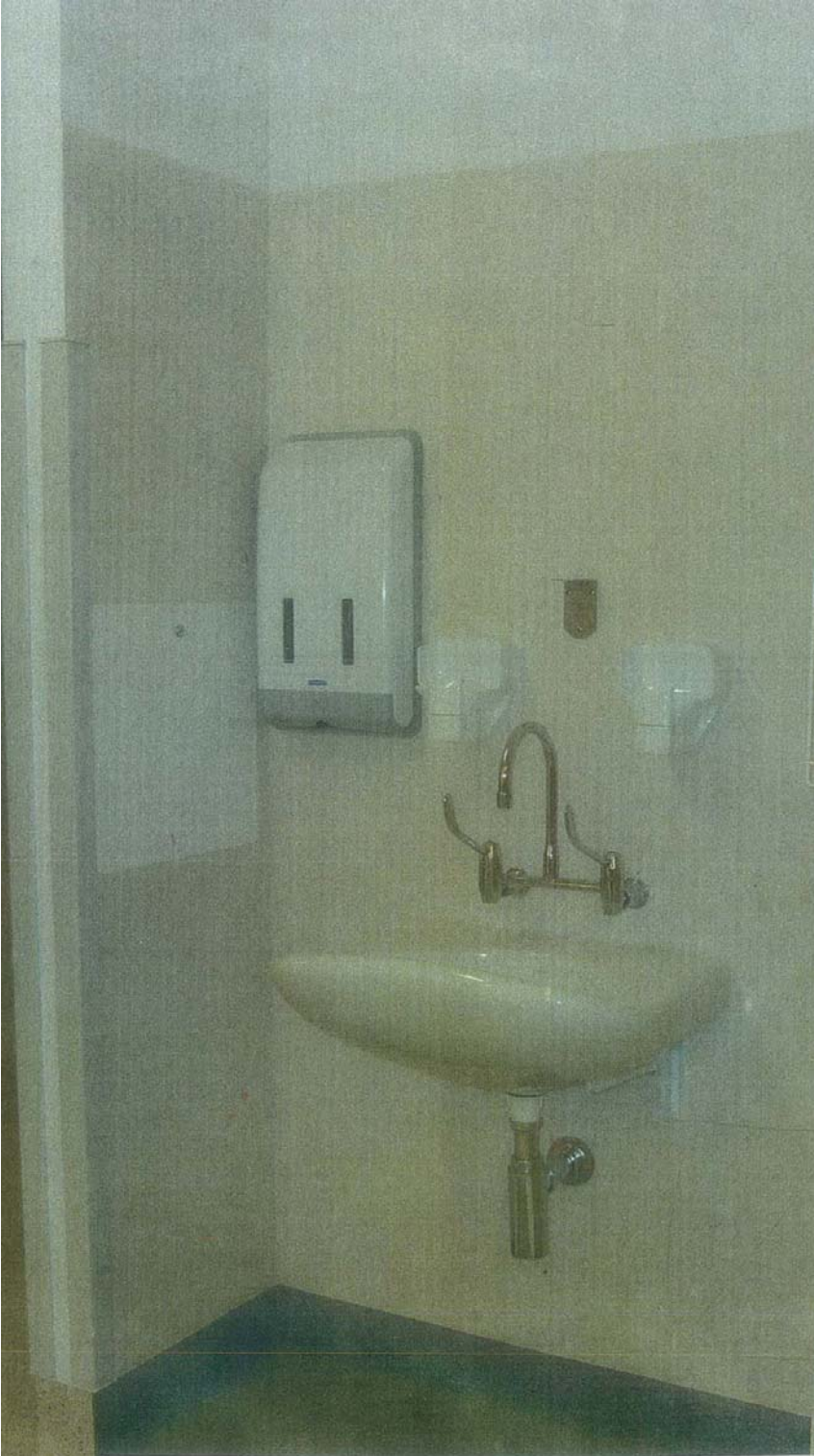
A typical hand rinse basin for staff use, as would be found in a hospital corridor alcove or treatment areas, the square white panel to the left of the basin is access to the thermostat bottle trap which will trap sharps and allow ease of removal, also the surgeons style elbow taps, these leave the basin clear of projections that impede cleaning, the taps have left hand operation, are quarter turn, ceramic seals are suitable for this arrangement because they tolerate the tap handles. This basin is cantilever bracketed from the wall to provide good cleaning and an arrangement requires structural consideration when fixed to a stud wall, or directly back to the other side of the wall. Unstable or careless users may use the basin for emergency situations, significant structural load
